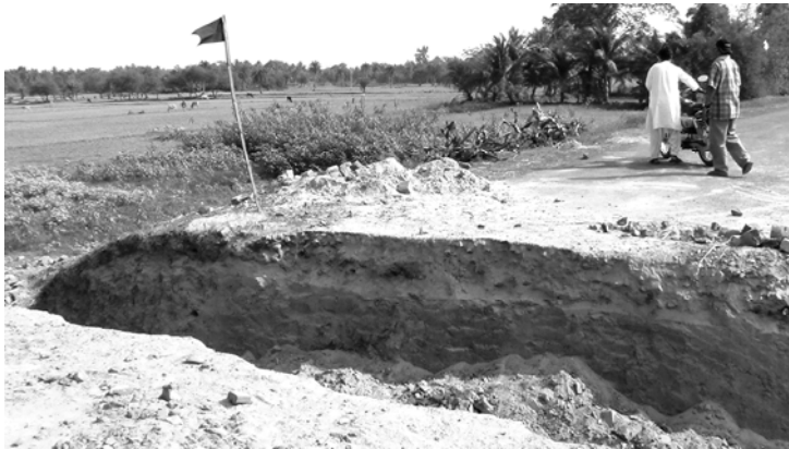
A trench on Prime Minister Village Road Project road, with a black flag of BUPC
